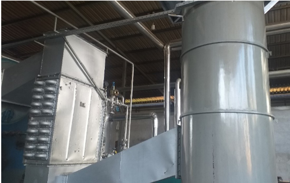
Figure 3a: Heat pipes of boiler
