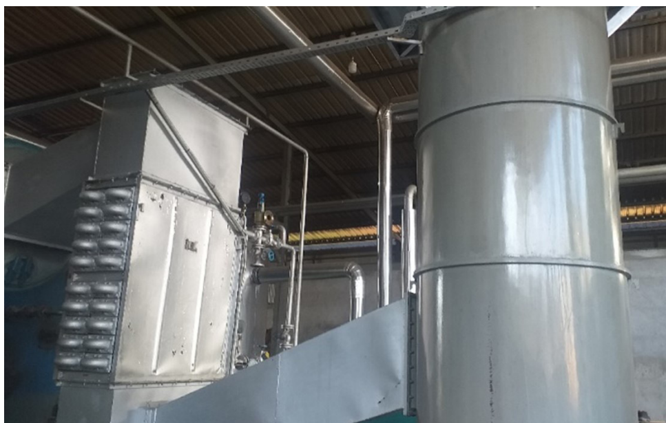
Figure 3a: Heat pipes of boiler
